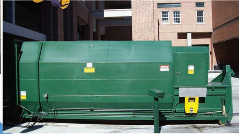
Self-contained Compactor Installation with Doghouse Hopper and Cart Tipper
